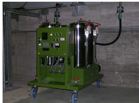
KLEENTEK ELC-R200SP-H installato su turbina a gas GE FR9FA.
